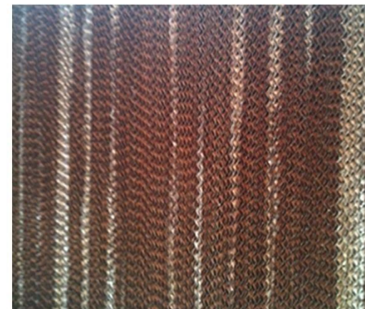
Evaporative cooling pad on June 25th, 2012
